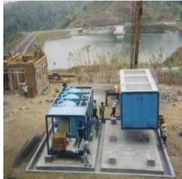
Kupang Project Water Treatment
