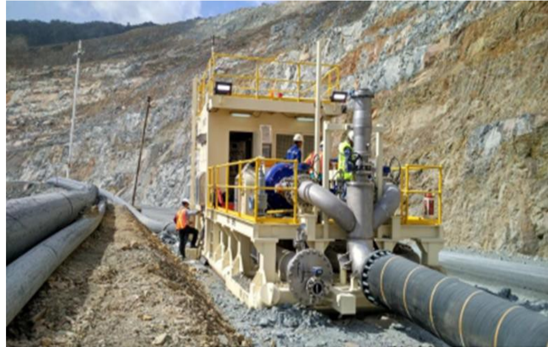
Newmont Dewatering Pump
